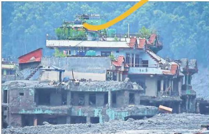
Damage in the aftermath of flash floods in Devighat in the Nuwakot district in Nepal on Thursday. (AP/PTI)
