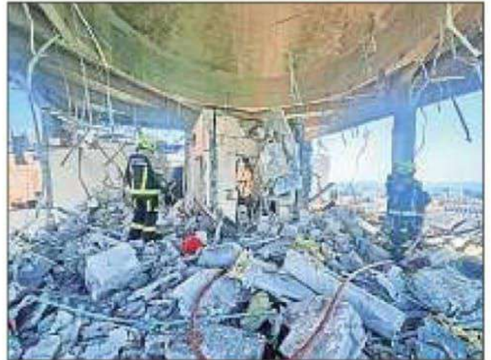
Bahrain civil defence and rescue personnel work in a residential building, which was hit by an Iranian drone on Sunday. (Reuters)
