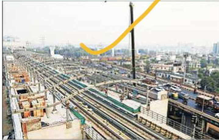
Work underway at Ahmedabad-Mumbai High-Speed Rail Bullet Train project near Bullet Train headquarters in Ahmedabad. (ANI)
