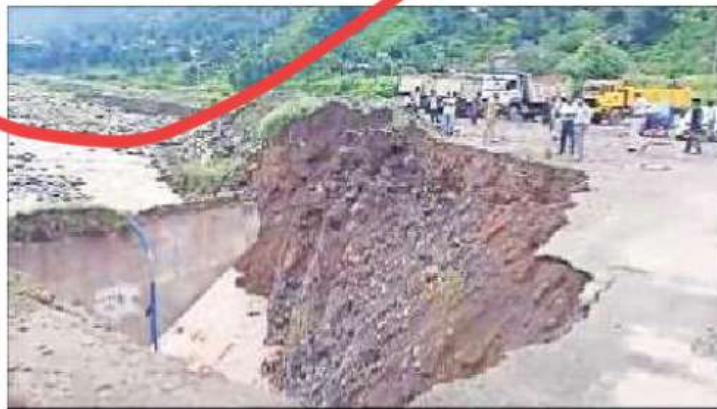
Part of Durangali Bridge washed away after heavy rainfall, in Poonch, Jammu & Kashmir on Sunday. (PTI)
