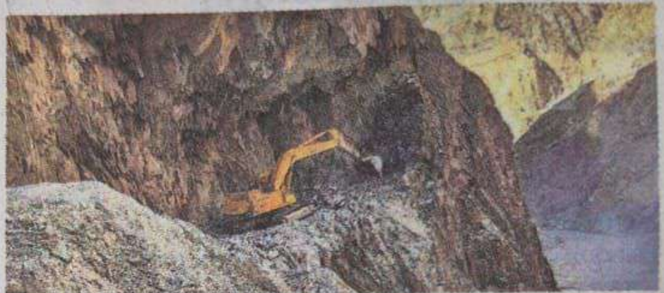
New avenues: Construction work of Shinku La tunnel under way near the Zaskar river in Ladakh. PTI
