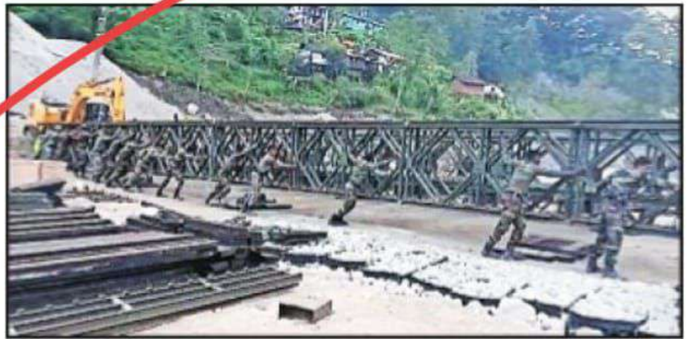
Troops of Indian Army's Trishakti Corps undertaking construction of Bailey Bridge over the Teesta river in North Sikkim on Sunday. (ANI)
